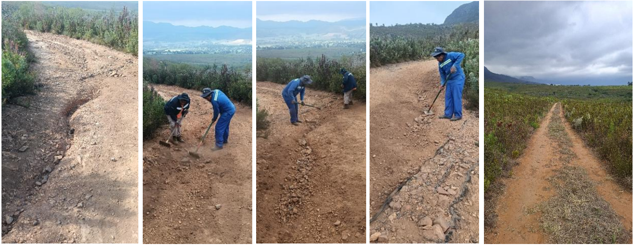
Figure 55: Water erosion damage on the reserve footpath. Figure 56 & 57: Staff grading the eroded path and clearing drainage lines. Figure 58 & 59: Stabilized path edges and newly maintained trail section.
