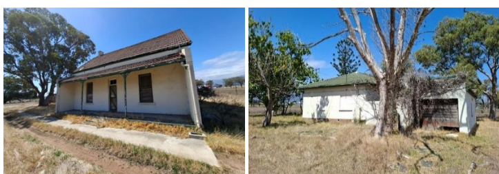
Figures 109 & 110: Buildings at Paardevlei due for urgent maintenance work
