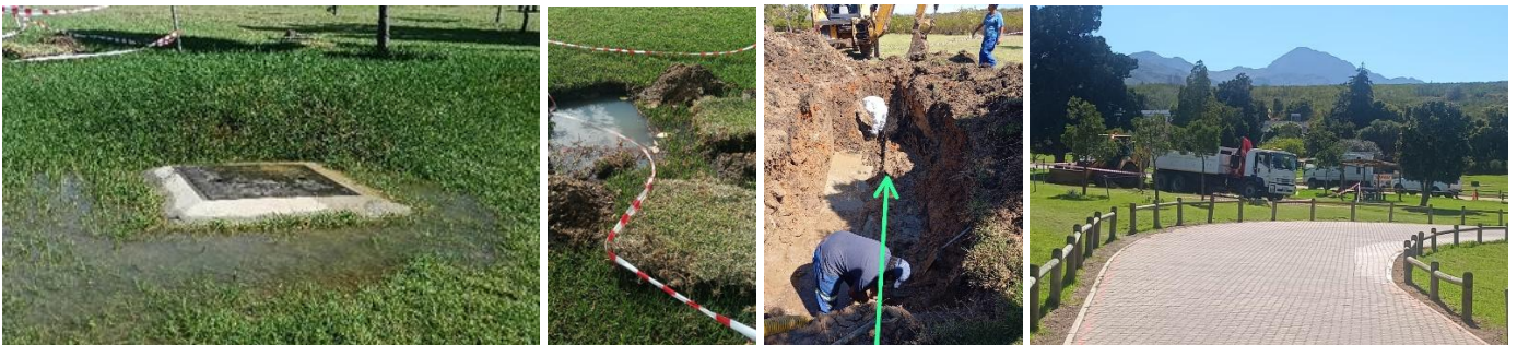
Figure 70 - 73: A burst water pipe at the Helderberg Nature Reserve picnic area and subsequent repairs.
