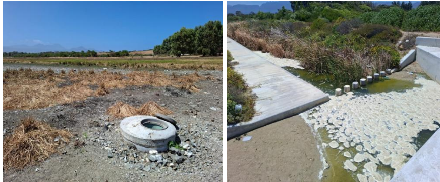
Figure 68 & 69: Observations following a sewer manhole overflow at Paardevlei canal
